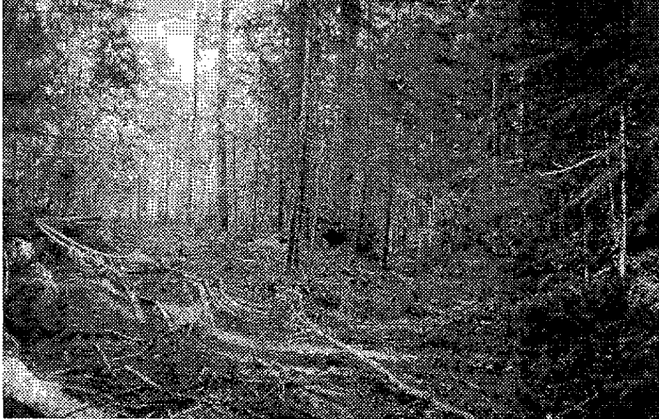
Figure 2. Before the channel was excavated, M&B cleared the channel right-of-way and selectively logged the nearby areas.
