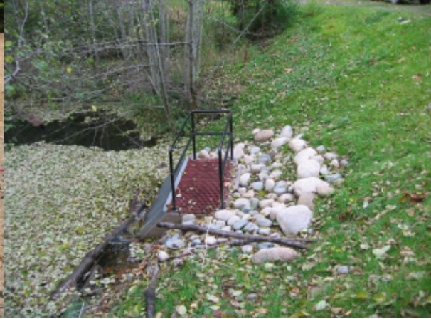
Figure 3 Trash Rack Complete
