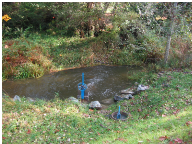
Figure 1 600mm Intake Valve and 300mm Bypass Valve
