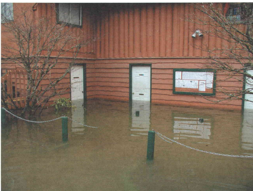
Photo 6. March 14, 2003. Approximately 24 hours after the peak of the flood. A building in the trailer park is flooded.
